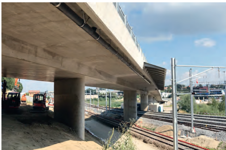
Fig. 2 Vue de la culée nord vers le sud. View from the north abutment towards the south.
